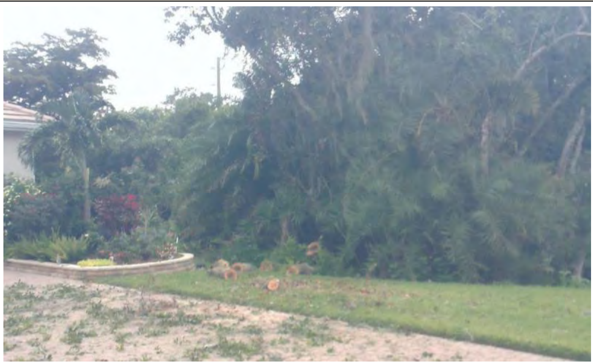
Removal of 2 diseased oak trees – one had fallen days earlier and the other tree leaned towards homeowner property. The oak had the ganoderma root rot disease. The price to cut down, remove and clean up was $650
